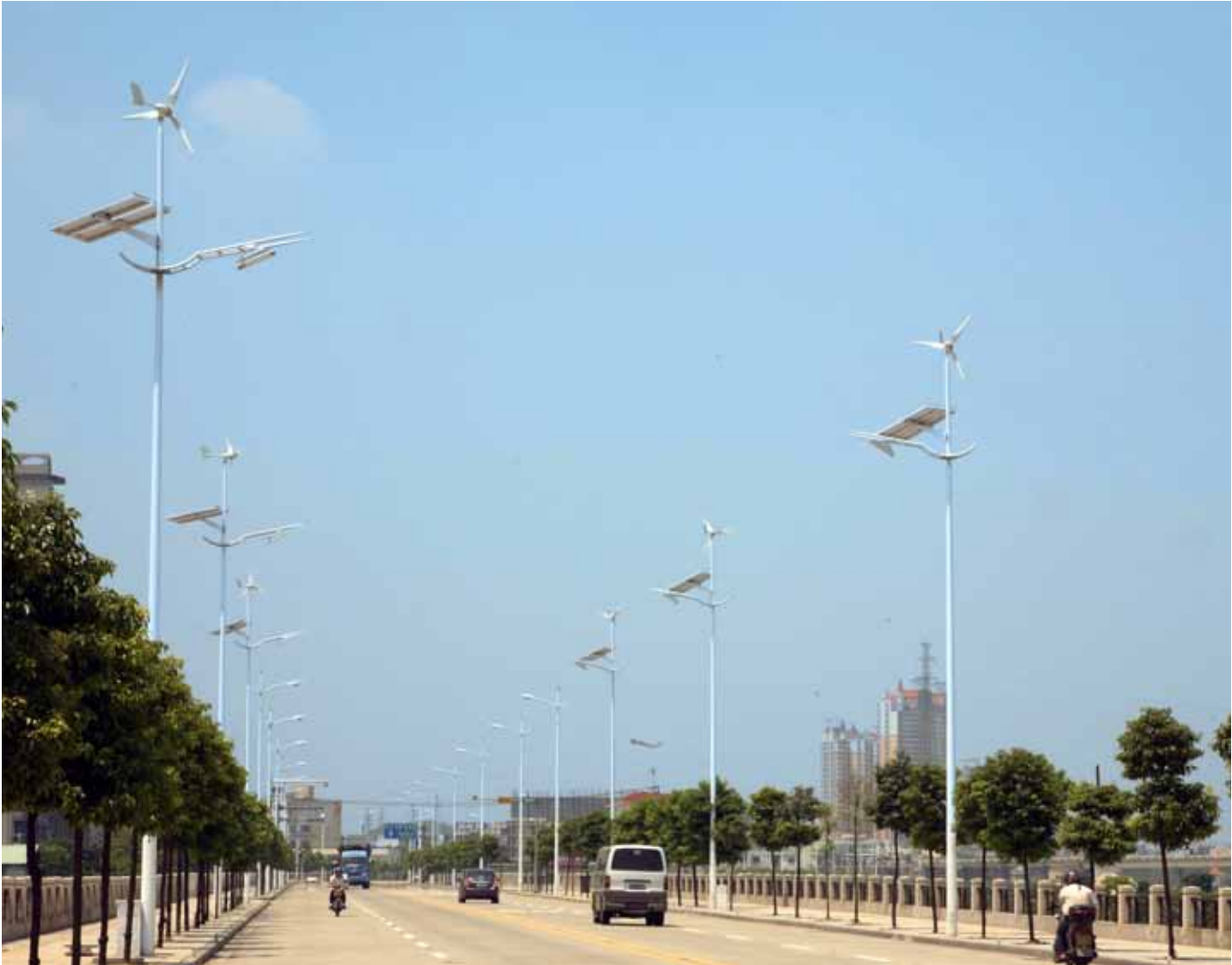
Wind-Solar powered LED street light in Shipai Wetland Park, Dongguan, China
